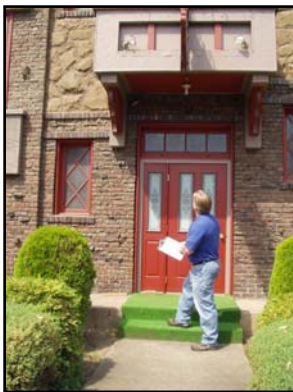
IHFA personnel inspect a Section 8 Voucher unit at Chateau Apartments in Lewiston.
